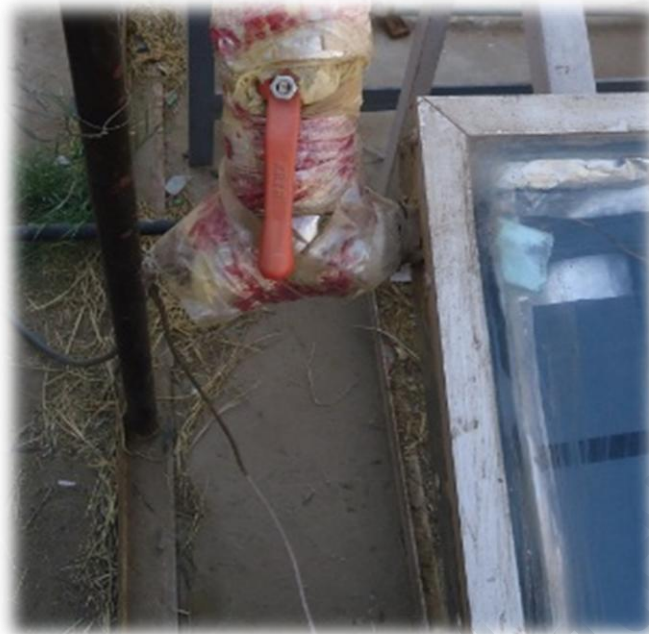
Fig 4.6 thermocouple at the collector outlet
